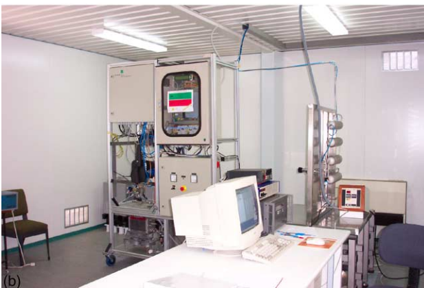
Fig. 2. Photographs of the outside (a) and inside (b) of the building hosting the solar hydrogen system.
